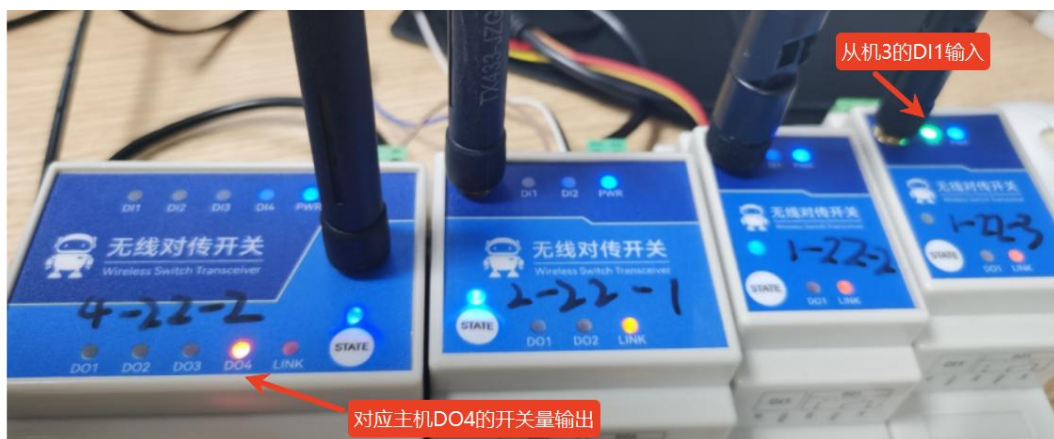
Figure 3-4-2 The switch input DI1 of slave 3 controls the switch output of the corresponding host D04 channel
